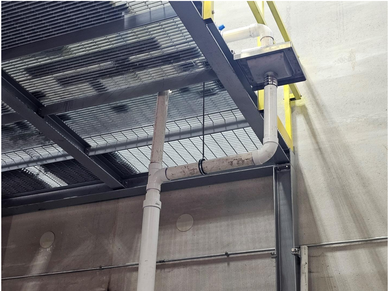
Figure 1 - Big - 750 Vent Stack
